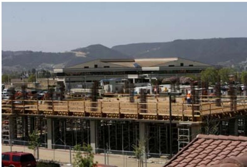
Ed Crisostomo / The Press-Enterprise Construction workers continue their labors on Rancho Springs Medical Center's expansion. The project is expected to more than double the size of the Murrieta hospital.
